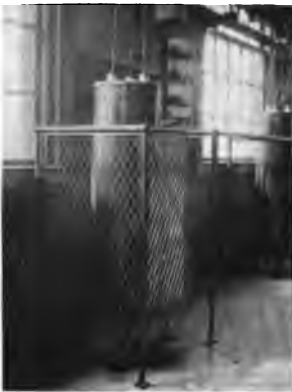
Fig. 4. Guards for Electrolytic Lightning Arresters, — 6600 Volts.
